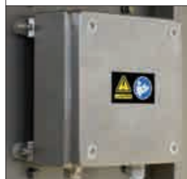
FIM enclosure box mounted onto the conveyor
